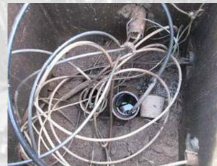
Manhole with 5,000V and 600V Cable (Asheville)
