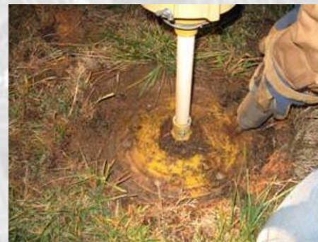
Rusted Base Plate
