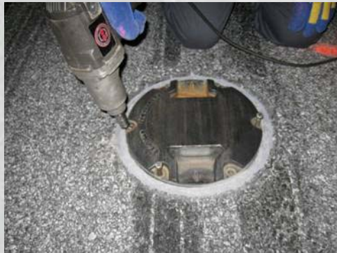
Existing Centerline Light
