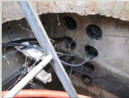
Manhole with 5,000V and 600V Cable (Per NEC)
