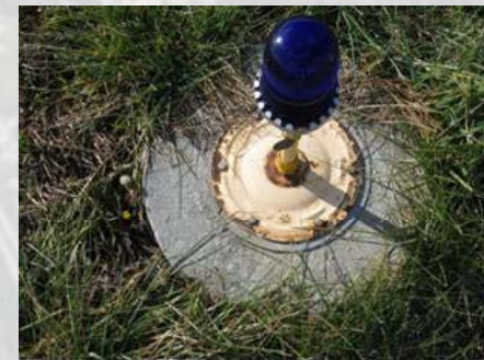
Rusted Base Plate
