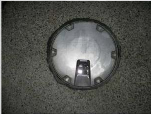
Existing TDZ Lights
