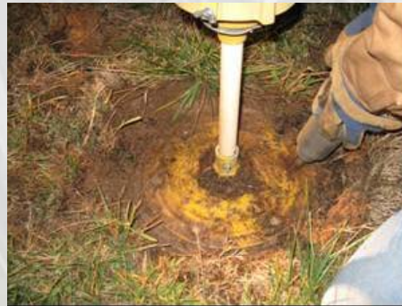
Rusted Base Plate
