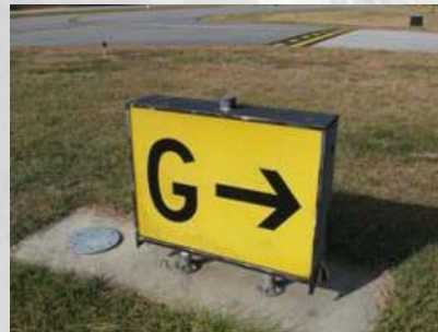
Runway Exit Sign (Cracked Panel)
