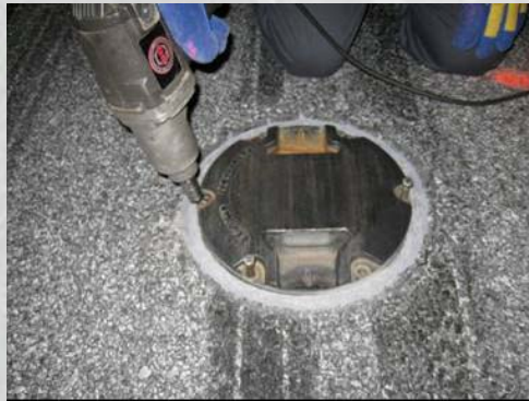
Existing Centerline Light
