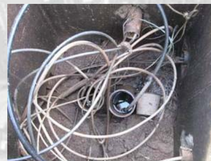
Manhole with 5,000V and 600V Cable (Asheville)
