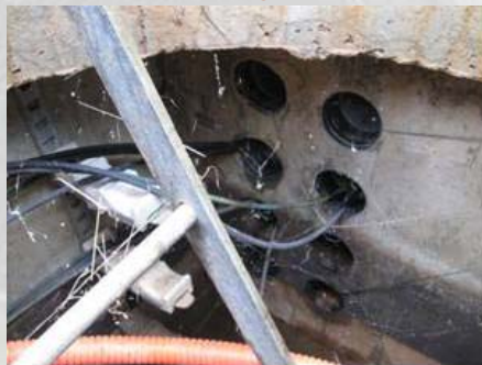
Manhole with 5,000V and 600V Cable (Per NEC)
